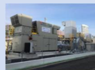
▲Hydrogen CGS demonstration plant
