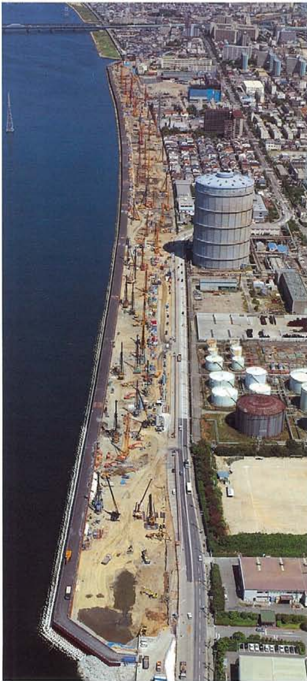
Ground improvement under way at the mouth of the Yodo River (September, 1995)
