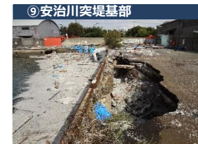
(岸壁補装陥没)
