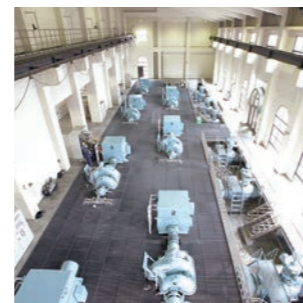
Kunijima Purification Plant
