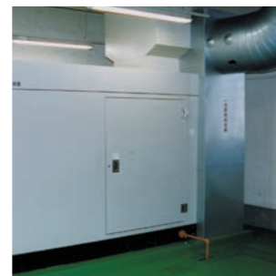
Sumiyoshi Distribution Plant (Non-utility generator for facility operation)
