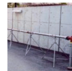
Temporary water taps
