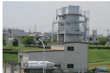
■ Figure: Granular active carbon injection equipment (Kuzuha Water Intake Facility)
