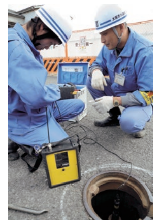
Water leakage investigation
