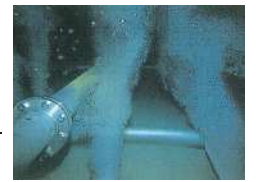
Ozone contact reservoir
